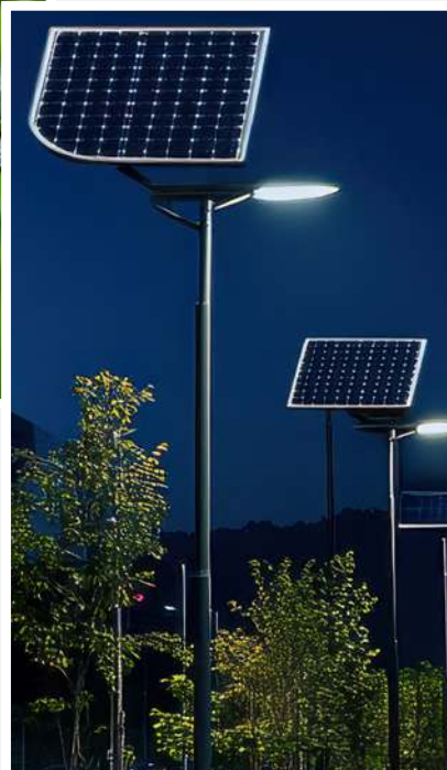
Solar lights of 45kW for common areas
